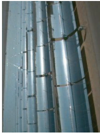
Figure 1: Rows of Thermal Collectors.
